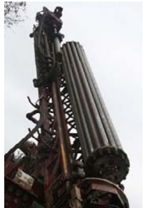
A 36-foot-tall drill was needed to install the geothermal system at the Gearon’s house in Derwood, Md.
